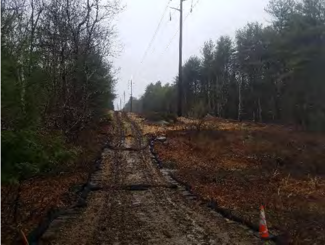
Fig 5: Access road between Strs 85-84, in wetland DW30. Mats need to be cleaned. Viewing west (05-01-20).
