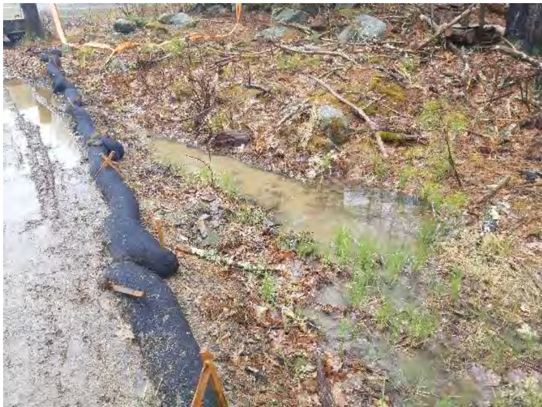
Fig 12: Turbid water entering culvert under access road to Str. 93. Wetland DW16. Viewing southeast. (05-01-20).
