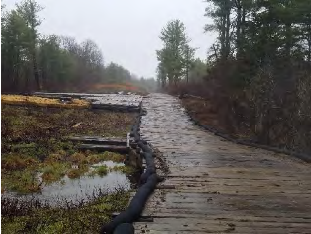
Fig 15: Bridge over stream DS60 in wetland DW58. Str. 44 work area in background Viewing north. (05-01-20).
