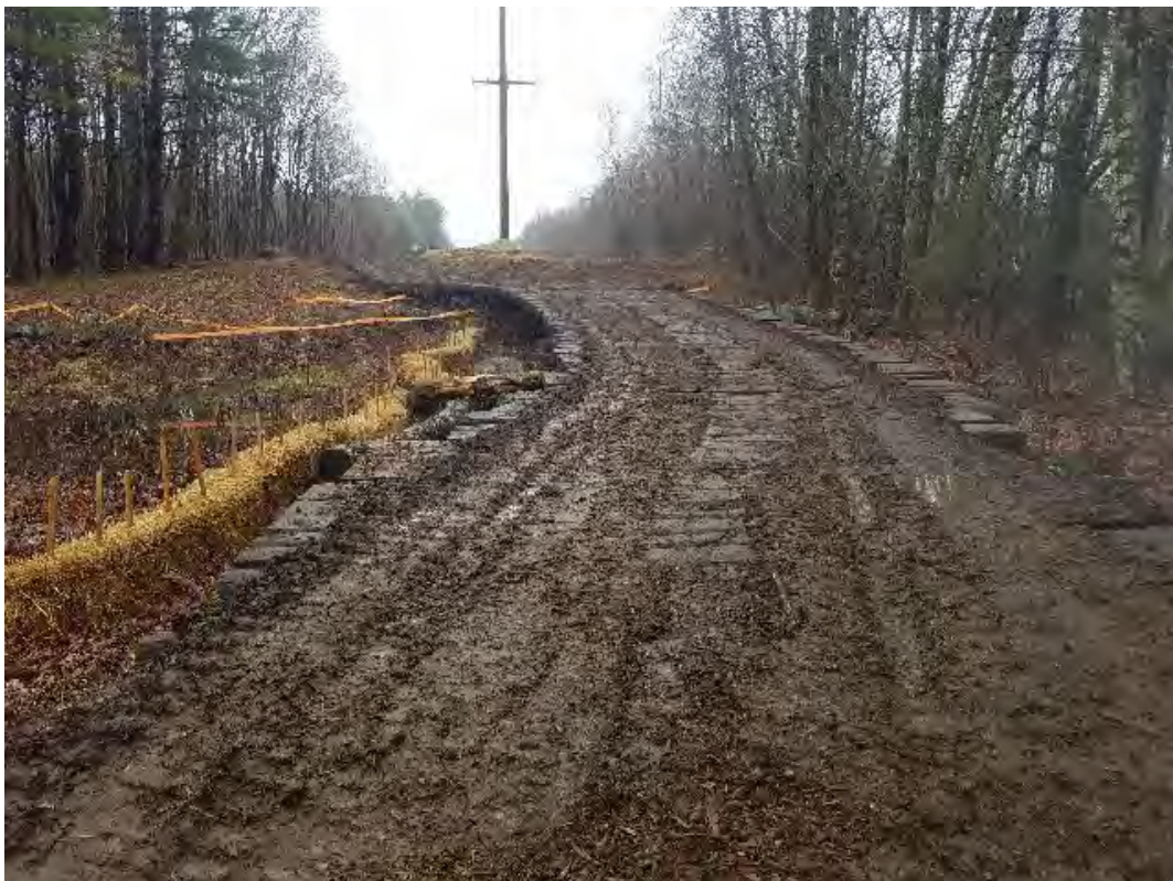
Fig 16: Access road adjacent to wetland DW43, between Strs. 36-37. Mats need to be cleaned. Viewing south. (05-01-20).
